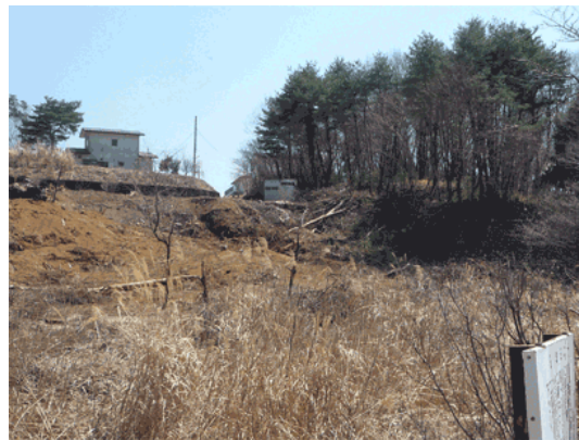
(c) 墓苑東斜面の崩壊 (西→東)
